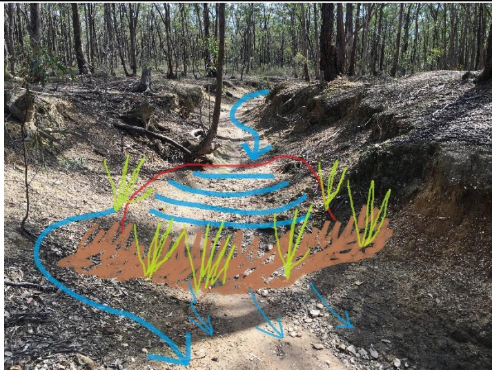
Image 1: Gully repair in a more incised section of watercourse below the old Soil Conservation Authority (concrete) structure. Annotations represent construction of numerous minor 'leaky weirs' from regrowth stems and local regolith, consolidated with robust perennial wetland tussocks ( Carex spp. etc.)
